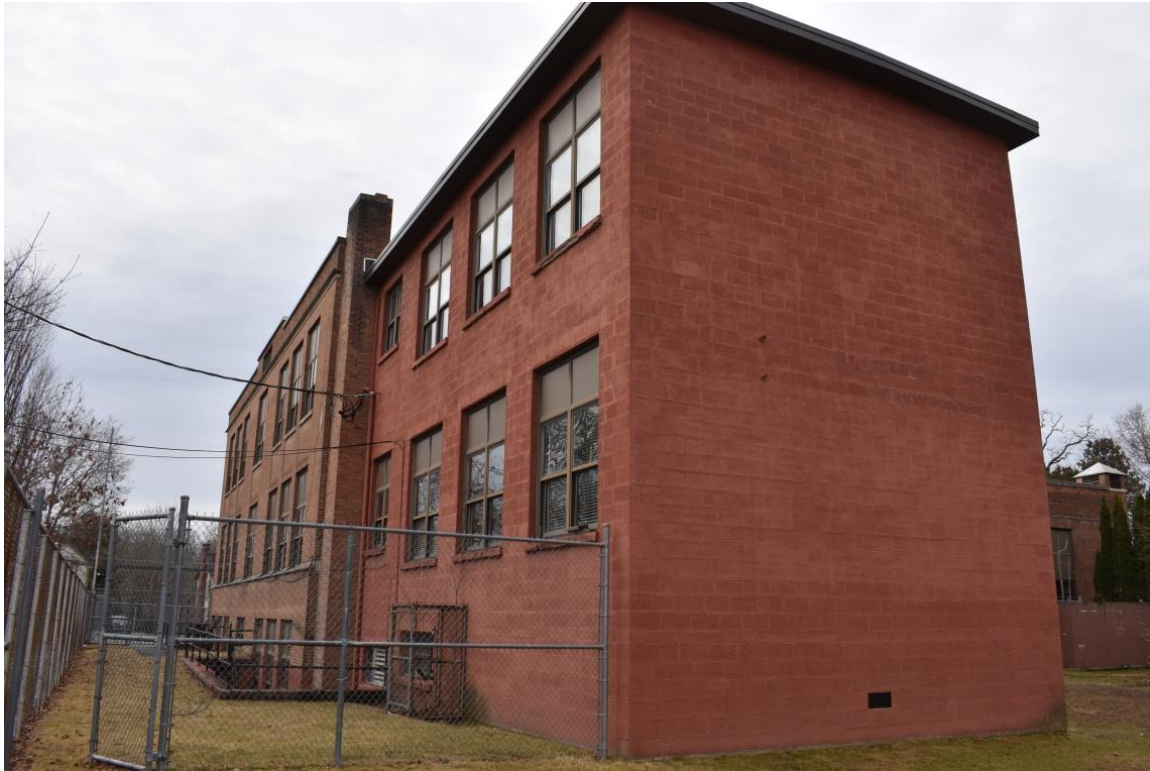
Photo 5: The northern side of the building is constructed of cinderblock, and painted red. View to the south.
