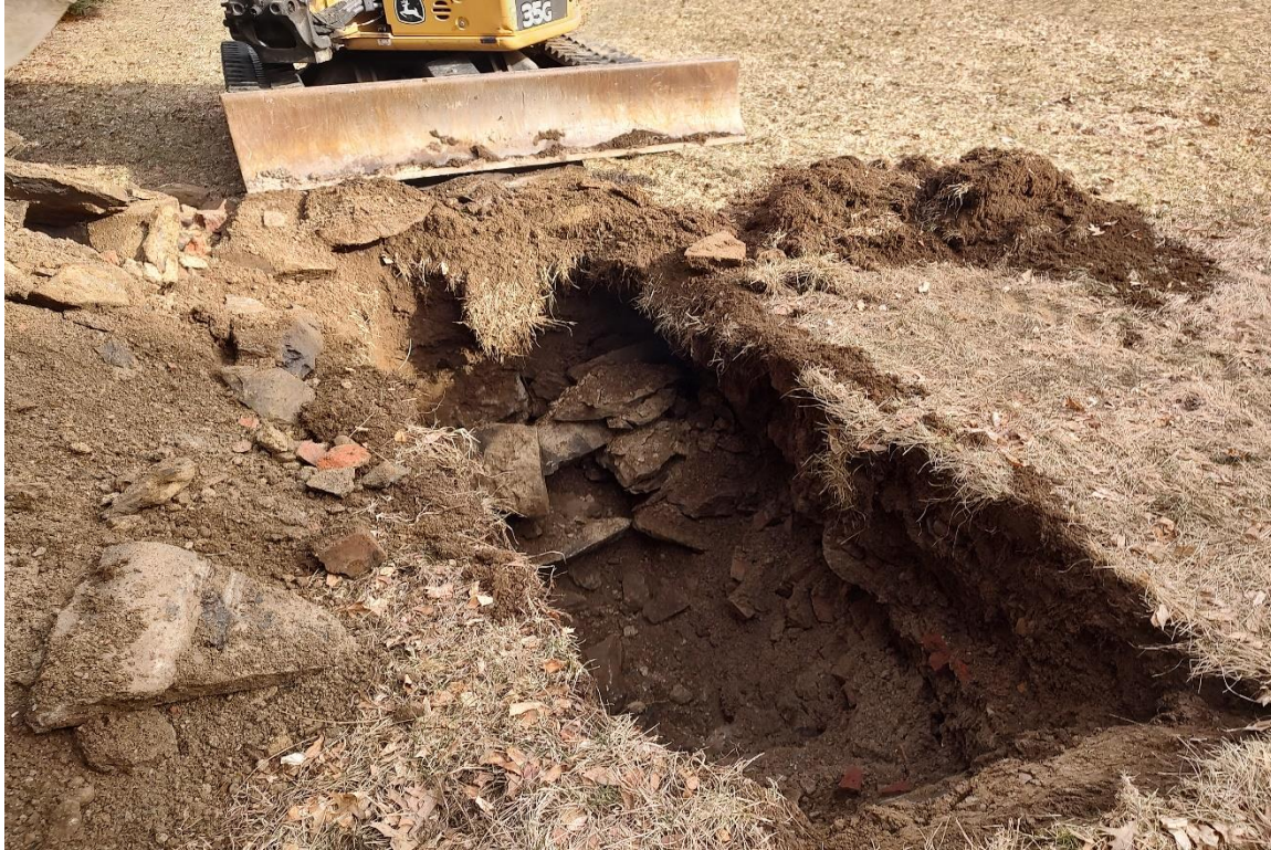
Photo 14: Deep tests, completed by the owner for proposed septic systems show extensive disturbance and building debris to the north of the school building.
